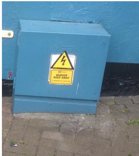
Figure 6 Warning Sign on Electricity Service Box in Stillorgan, Monolingual English
